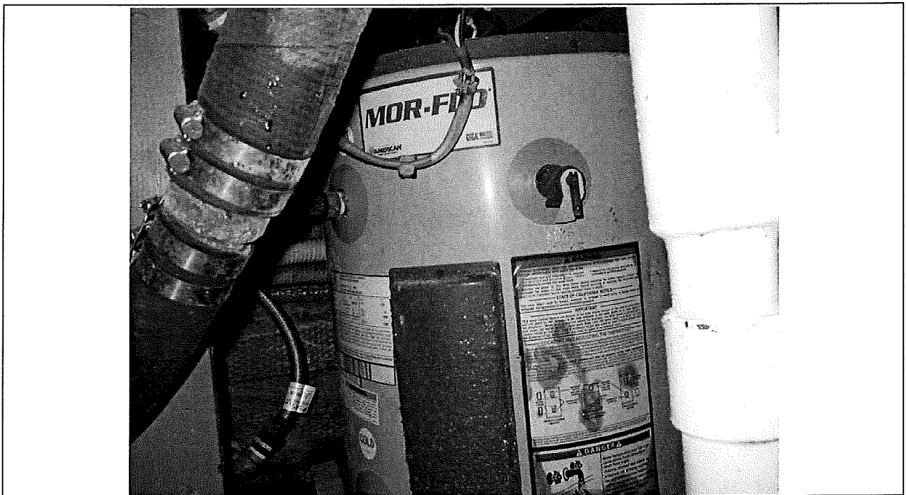
HOT WATER HEATER
