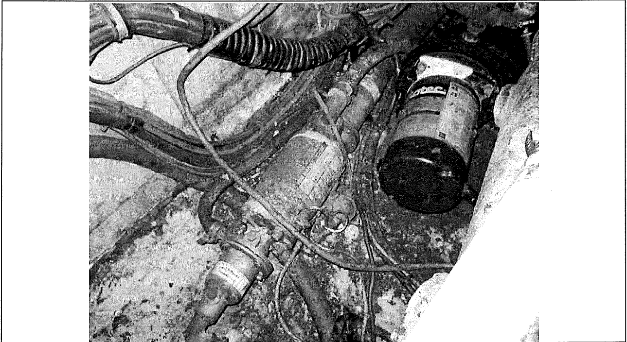
MID HEAD PUMP AND AIR CONDITIONING RAW WATER PUMP
