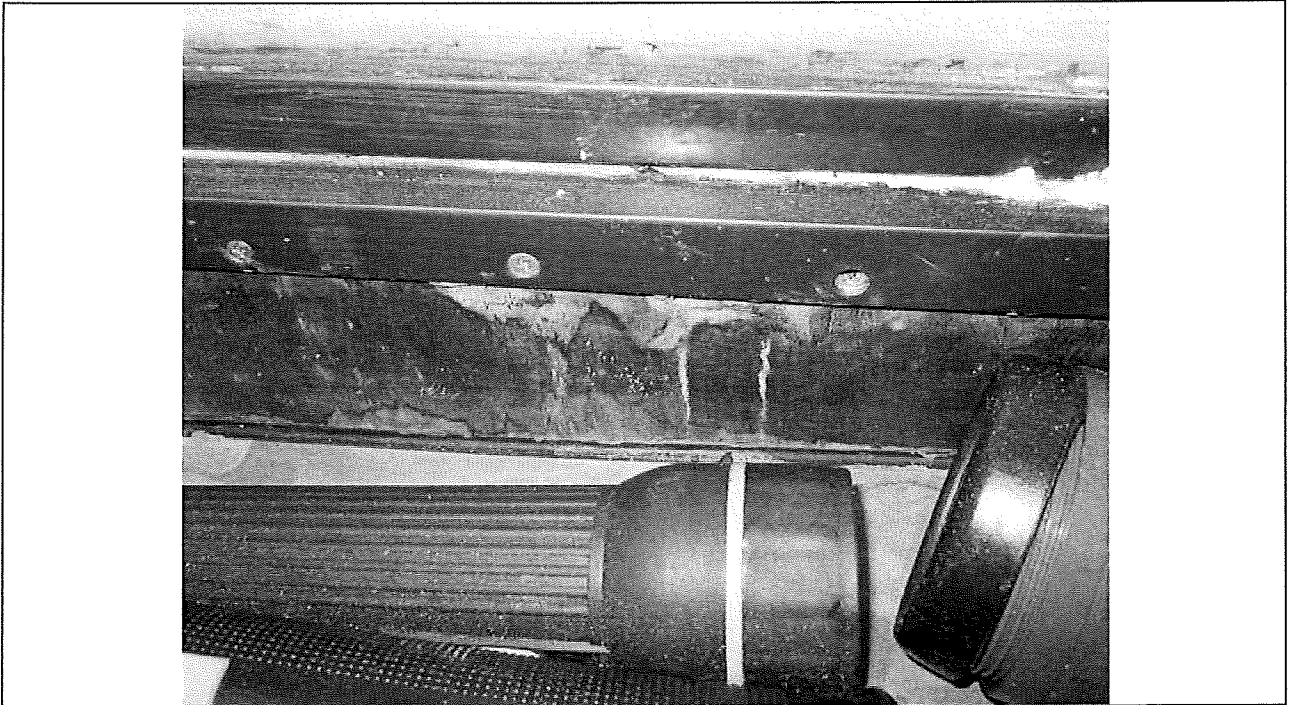
INDICATIVE OF WATER INTRUSION DAMAGE AT WINDOW FRAMES
