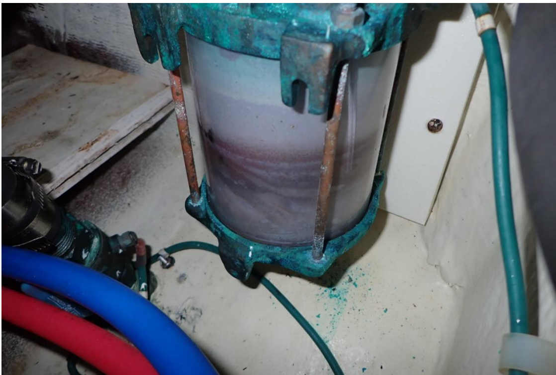
13. Generator seastrainer fouled
