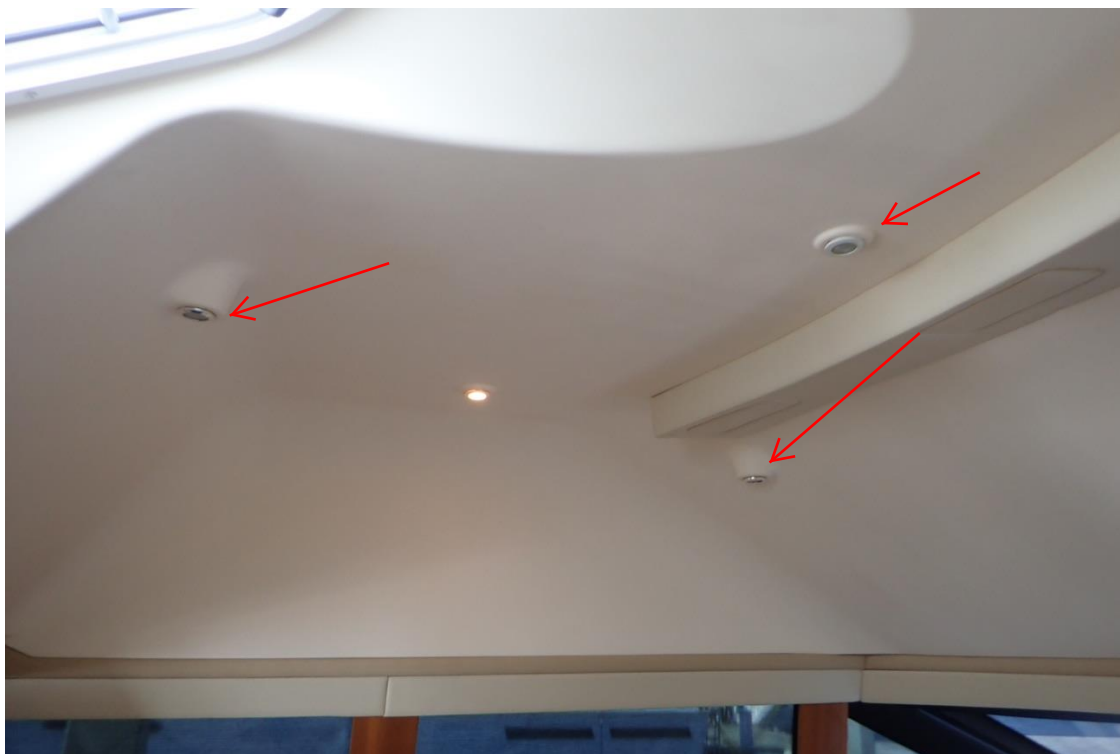
40. Lights inoperable at lounge
