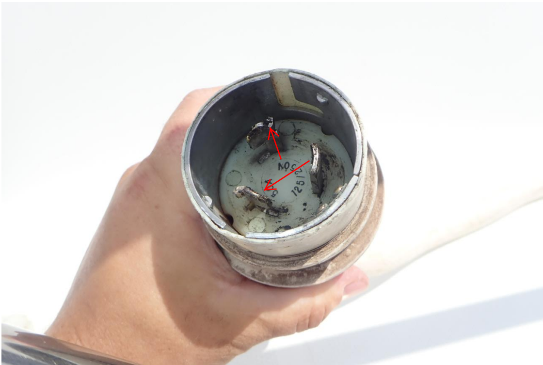
49. Arc damage to shore cable
