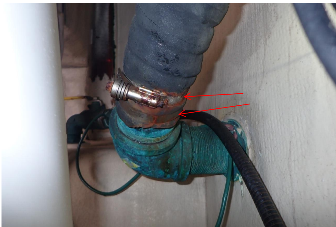
32. Broken and corroded clamps at generator exhaust in port lazarette
