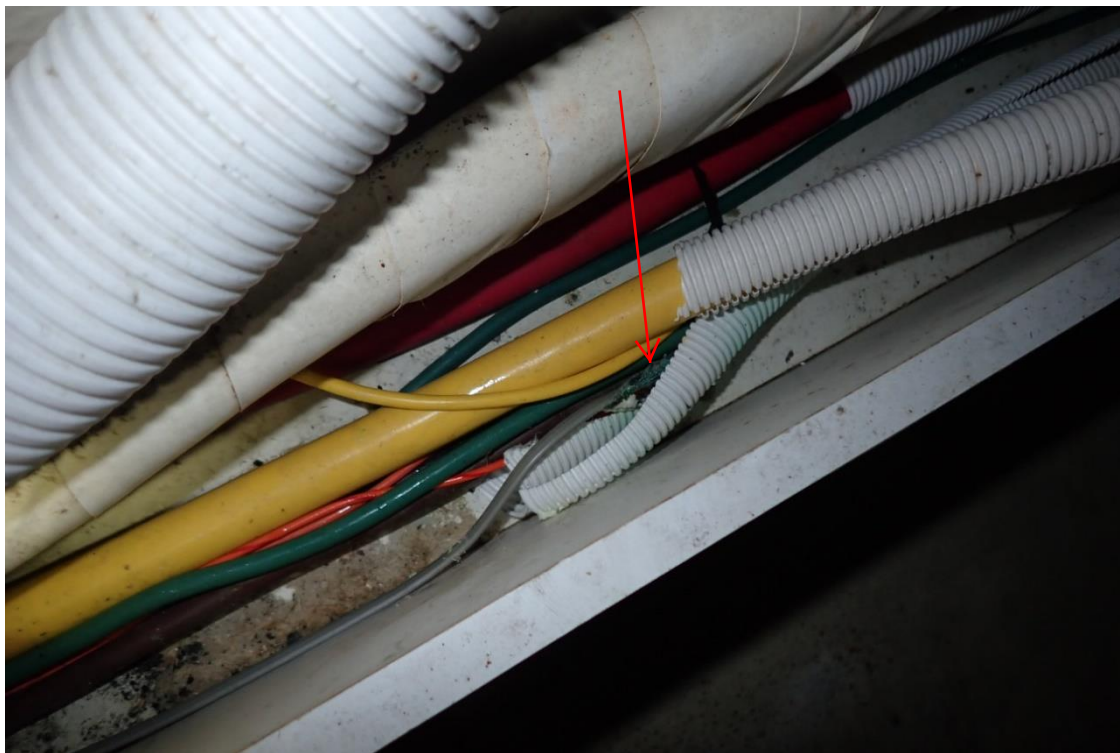
21. Overheating damage to wiring at starboard aft lazarette
