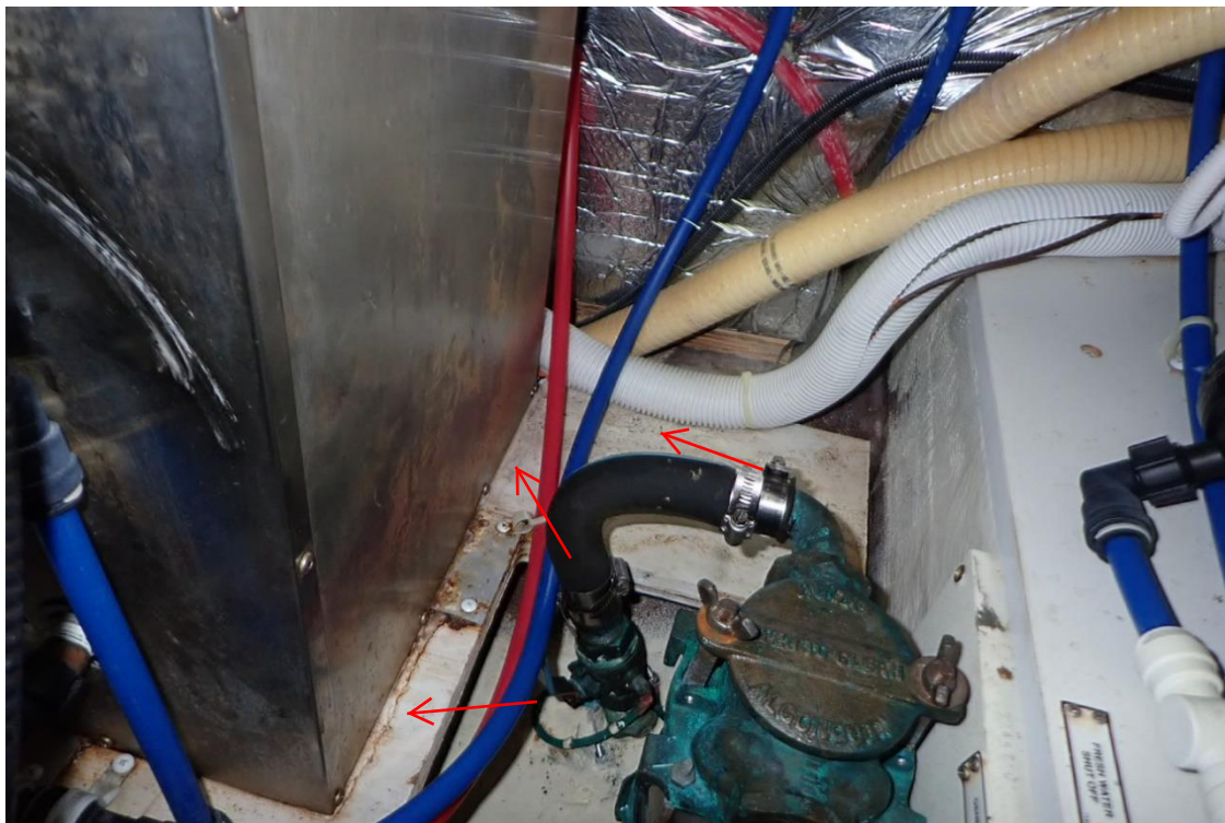
11. Standing water from apparent leak at water heater shelf
