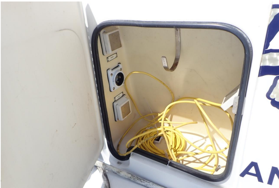
47. Shore power inlets
