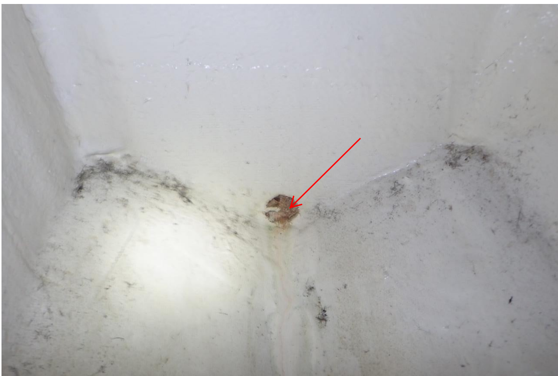
42. Forward limber hole fouled, centerline
