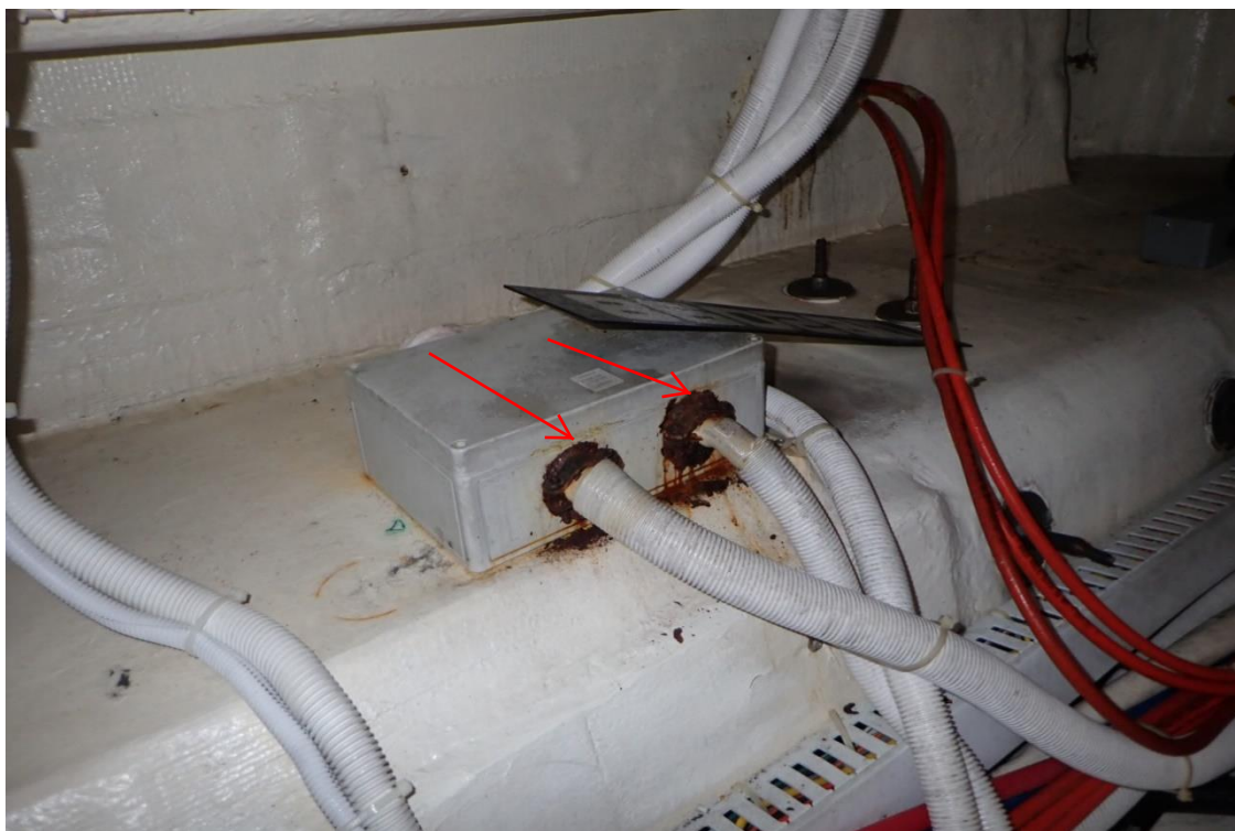
26. Corrosion at junction box in aft lazarette
