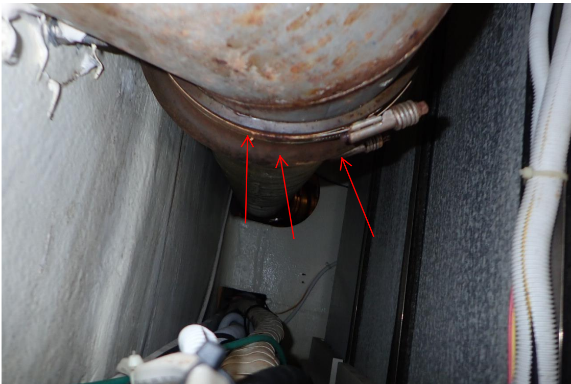
33. Corroded clamps at port exhaust fitting at port lazarette
