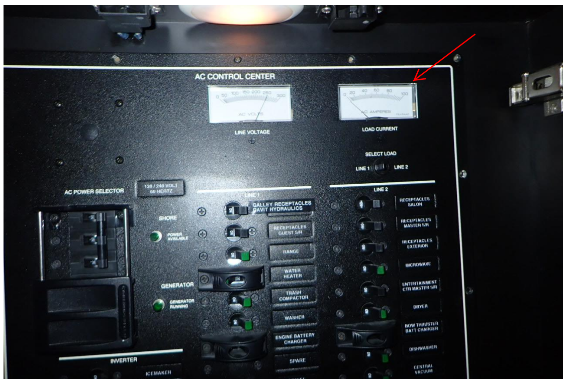
39. Ammeter not operable
