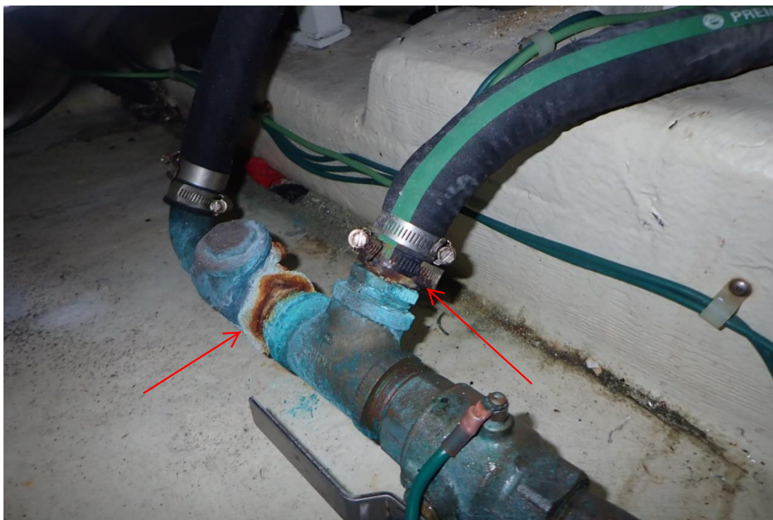
22. Broken clamp, corroded fittings, and leaks at air conditioner raw water intake
