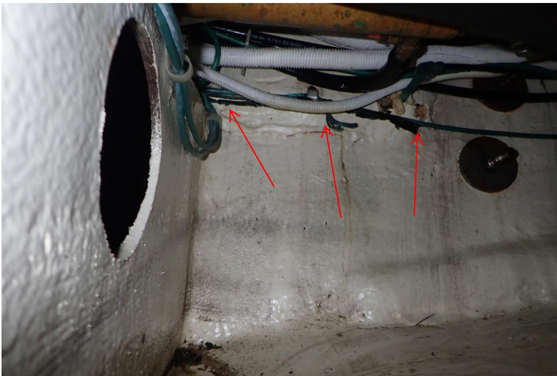
29. Damaged wiring from prior overheating
