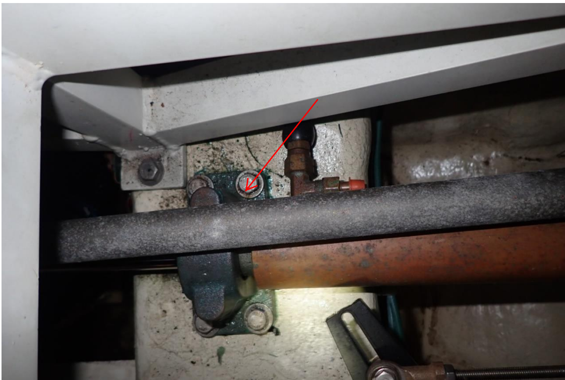
28. Steering fluid leak
